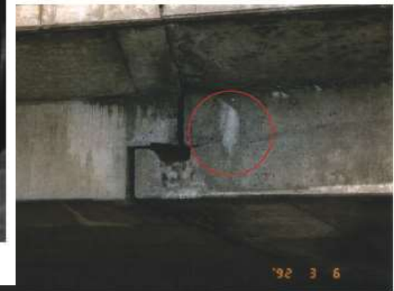
Figure 4.3 Concrete degradation on the east abutment of the de la Concorde overpass in 1992 a) North lateral face 29 b) South lateral face 30
