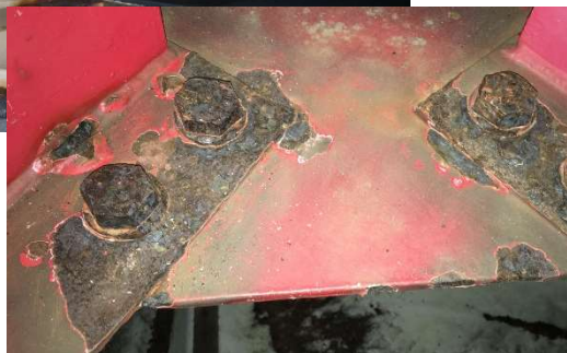
鋼桁の腐食 Corrosion in steel girder
