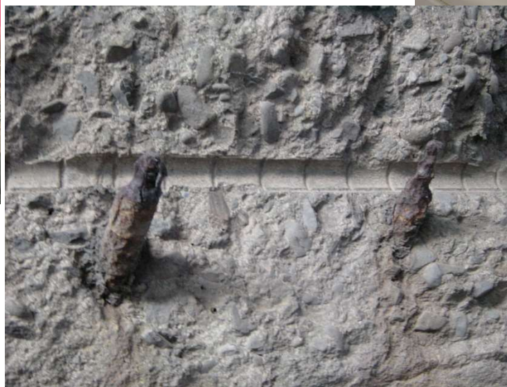
鉄筋の腐食 Corrosion of reinforcing bar
