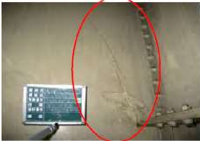
鋼桁の疲労亀裂 Fatigue crack in steel girder
