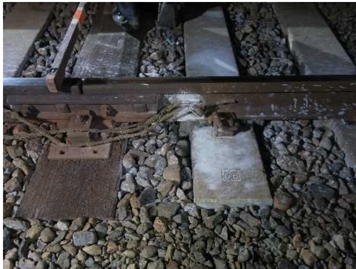
Fouled ballasted track in aged existing line
