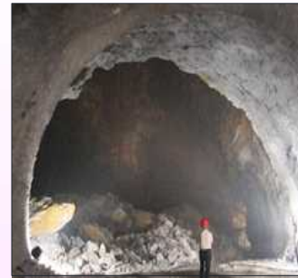
(2) 隧道塌方冒顶
