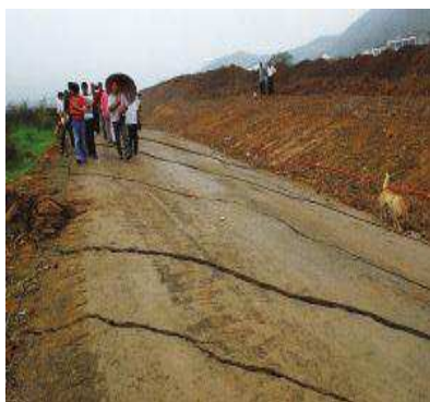
施工期间路基失稳破坏 Instability failure during construction process
