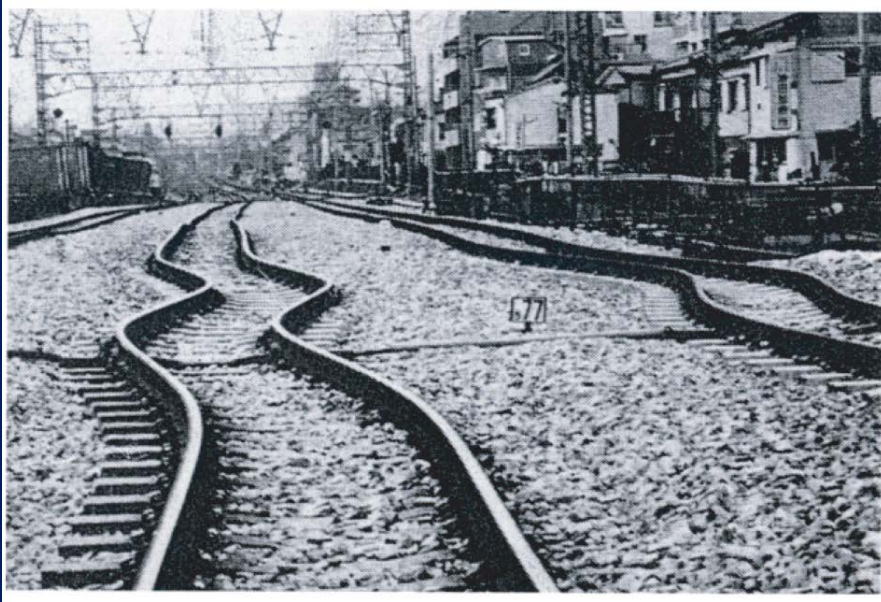
Damage observed after an earthquake (Momoya et al. 2013)
