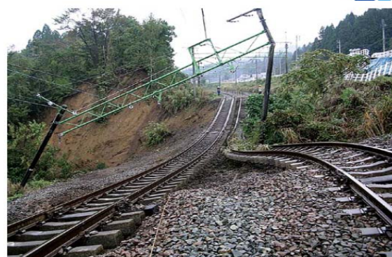
Damage case of embankment in the 2004 Niigata-ken Chuetsu Earthquake
