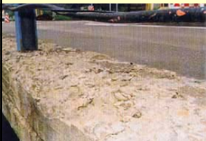
Result: Breaking-up and structural damage
