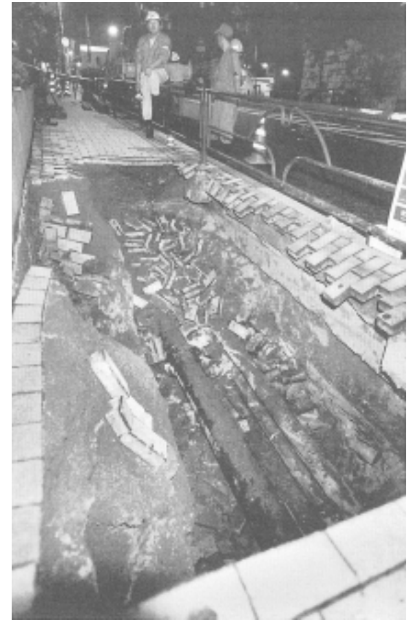
Road sinking at Isarago in Tokyo
