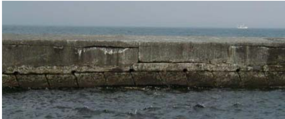
Bigger damage for later constructed part
