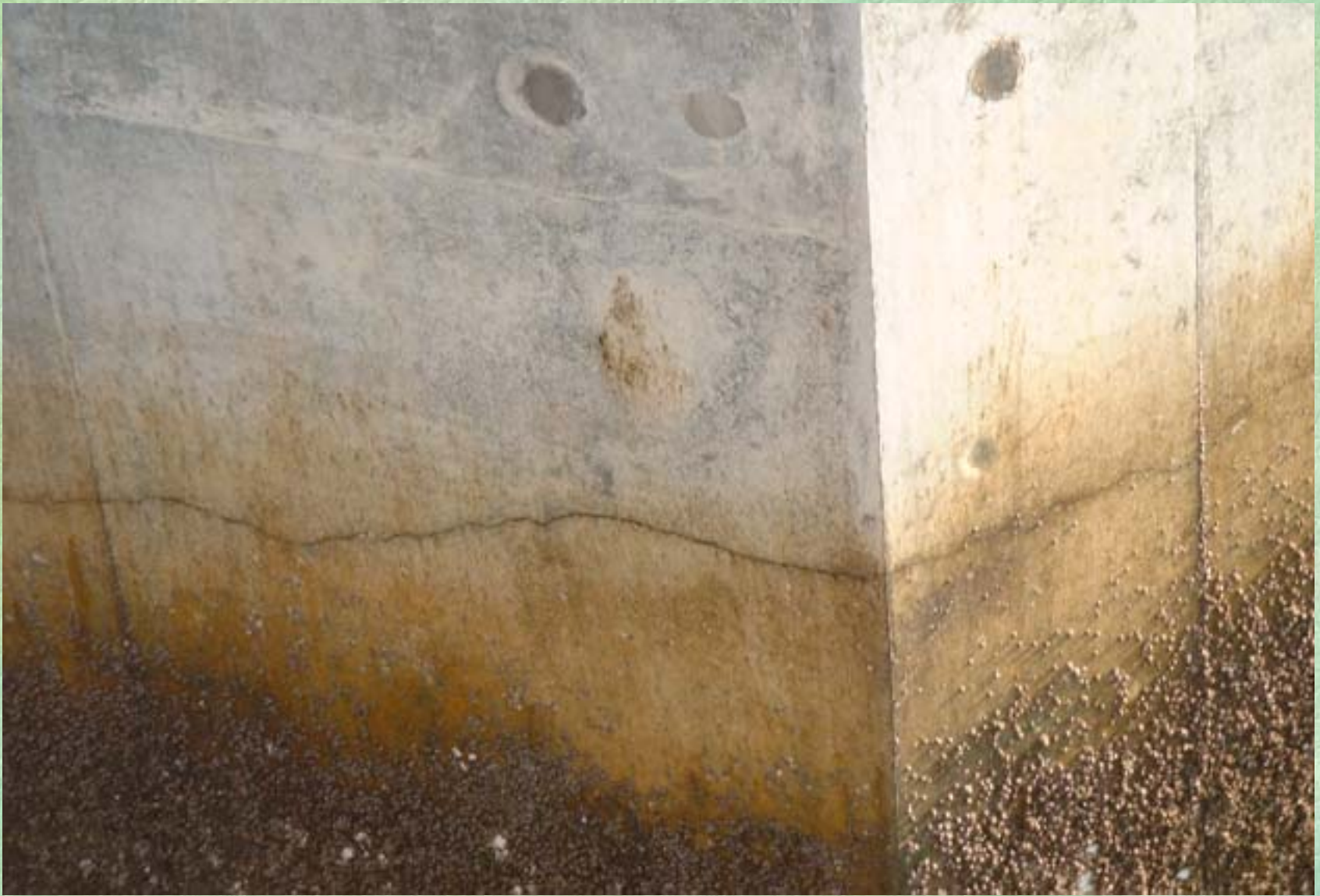
Appearance of Thermal Crack on the Pier
